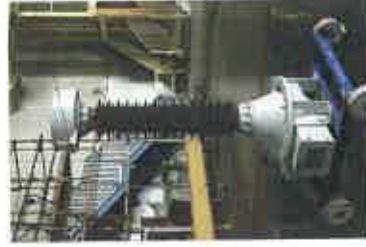
Fig. 4 Wet test of voltage transformers type PV 123 at power frequency voltage 50 Hz.
